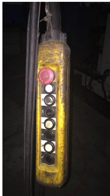
Figure 1.2 Manual remote control hoist crane in Mitra Adyaniaga.PT, the manufacture of boilers, Surabaya - Indonesia
